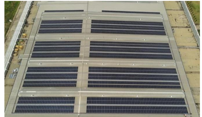
Thailand (2) ▶ Installed solar system under PPA
