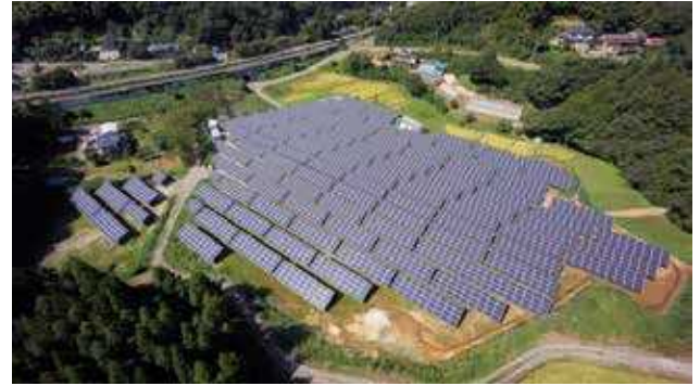
Miyagi Shiraiishi 1003 kW
